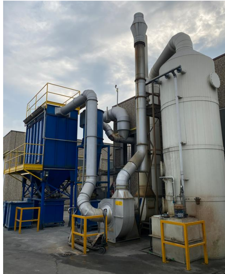
Off-gas treatment to remove dust, fume and acidic emissions
